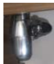
Wash basin pipe siphon
