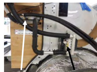
Heat exchanger, booster
