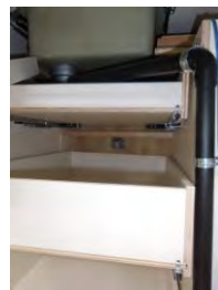
Sink screw siphon
