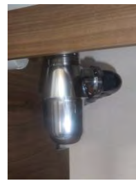
Wash basin pipe siphon
