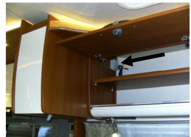
Distribution box near TV cupboard
